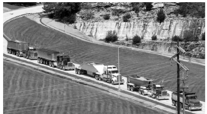
Dump trucks of many types line State Route J near Clarence Cannon Dam in June. The rock they carried was used to form a protective wall around the dam's substation. (Photo by David Cheek, Mark Twain Regional Council of Governments)
